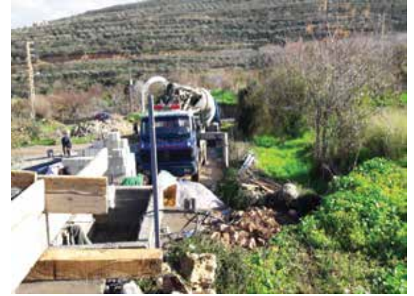
Pumping Station Lebanon 2018
