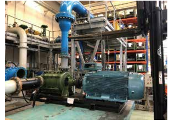
Factory Pumping Test 640 KW Italy 2018
