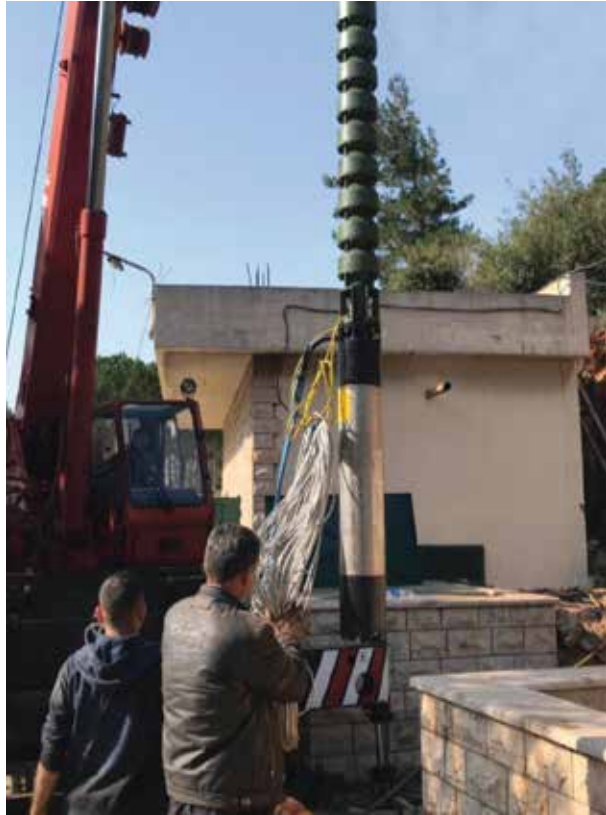
Solar Pumping Station (Pump Capacity 100 CM/hr) Lebanon 2021
