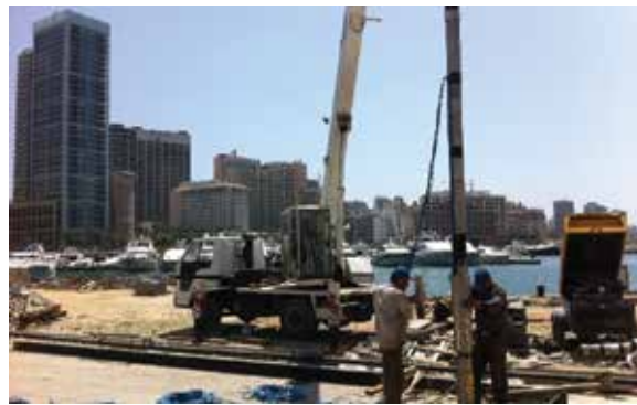
Sea Water Intake Wells For Condenser Cooling Lebanon 2010
