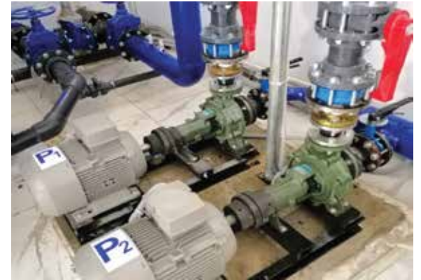
Pumping Station Lebanon 2019
